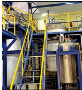
The bioreactor at IIT-Kharagpur that produces hydrogen from distillery effluent
